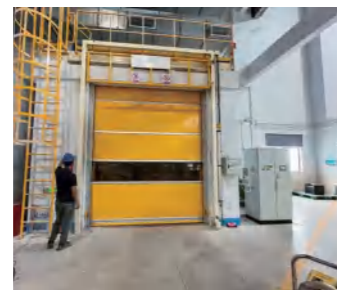
Freight elevator interlocked high speed door
