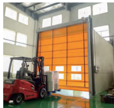
Geomagnetic induction buffer room stacking high speed door
