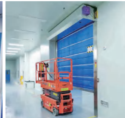
Inorganic cloth fire doors in clean areas
