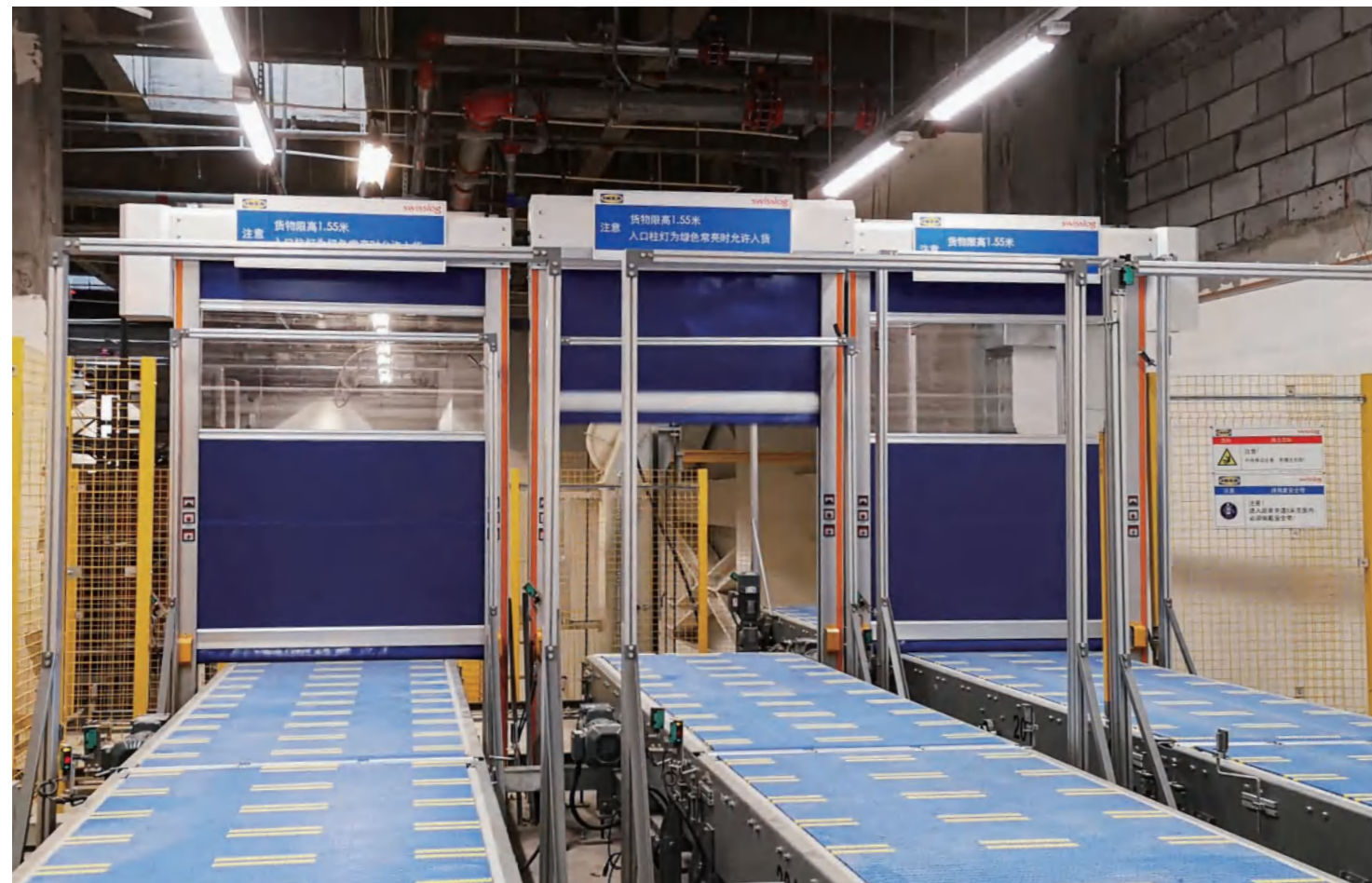
Conveyor belt linked high speed door (IKEA)
