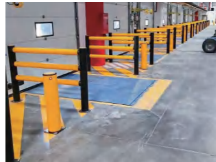
Protective barrels for building columns
