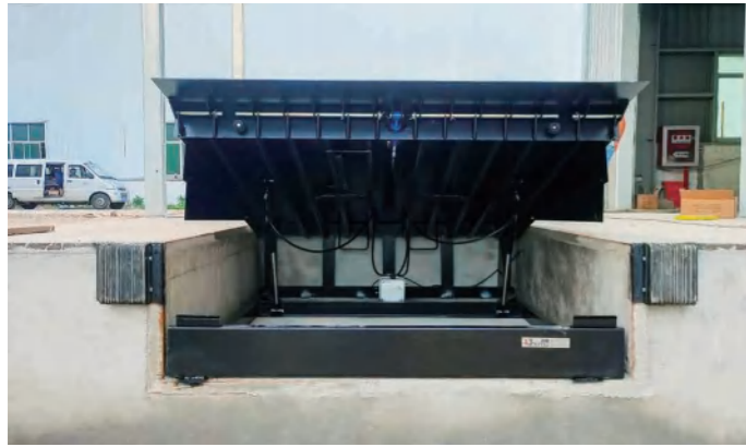
Standard loading and dock leveler
